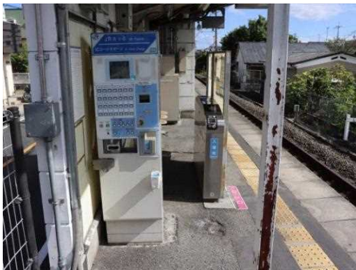
舗装面の凹凸
